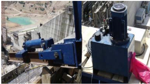
Fig. 16. Hydraulic jack (a), electromotor for electric pump (b).
