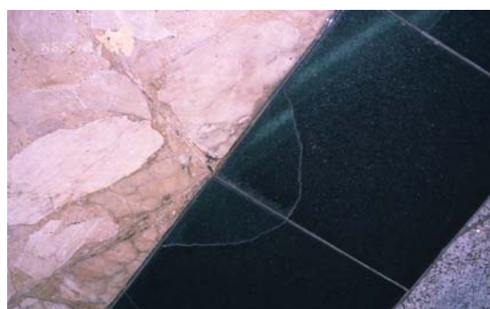
Fig. 2. Crack in cladding stone. Probable cause: a deficiency in the distribution of the mortar of settlement.
