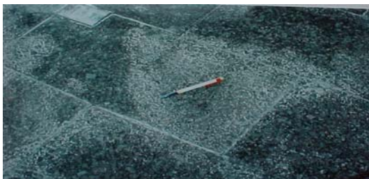
Fig. 7. Manifestation of mineralogical alteration of stone and occurrence of efflorescence. floor of the foyer building located at 3a. avenue, lined with granite coffee Bahia.
