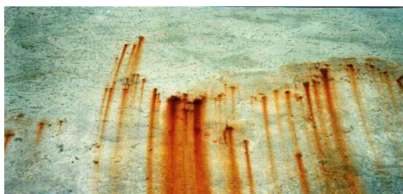
Fig. 5. Granite showing stains. Probable cause: oxidation of pyrites.
