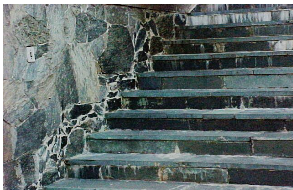
Fig. 1. Spots and efflorescence on the surface of the stone coating distributed slate. Residential building stairway, with approximately 5 years, in the city of São Paulo. Probable cause: excess water of kneading of the mortar.
