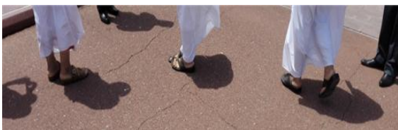
Fig. 2. Examples of the surface conditions observed in the affected pavement Sections.
